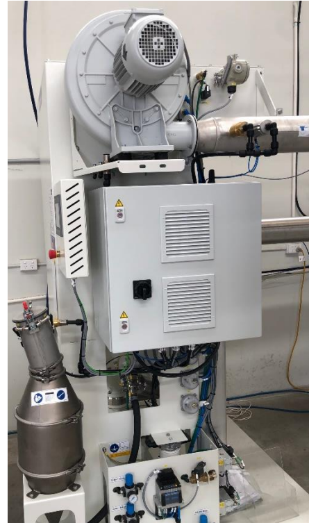
Figure 1: Fully Installed Fume Extraction Unit
